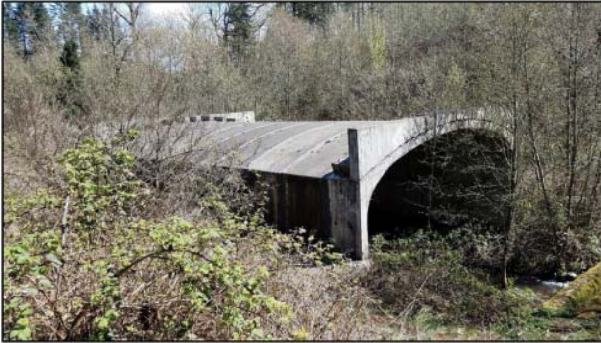
Box culvert over Jory Creek at southern terminus of Lone Oak Road, near Muirfield Avenue
