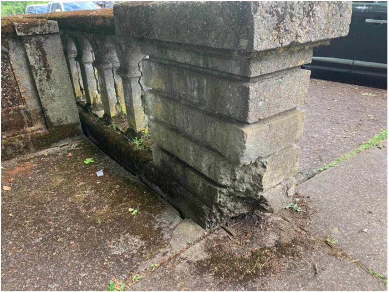
The railings on Liberty St. are basically in the same poor condition:
