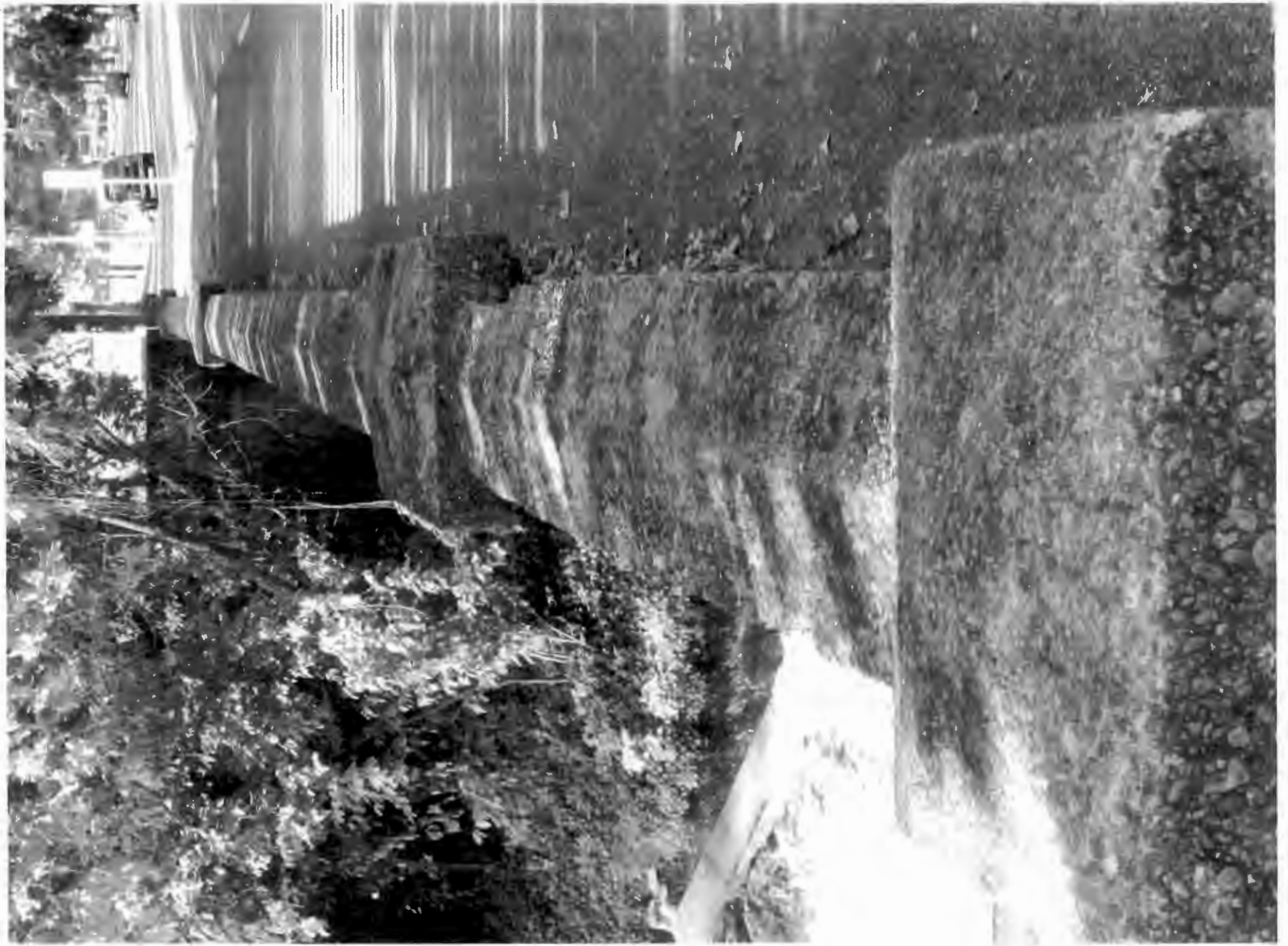
Biological growth on the bridge rail in the shadow of overgrown vegetation
