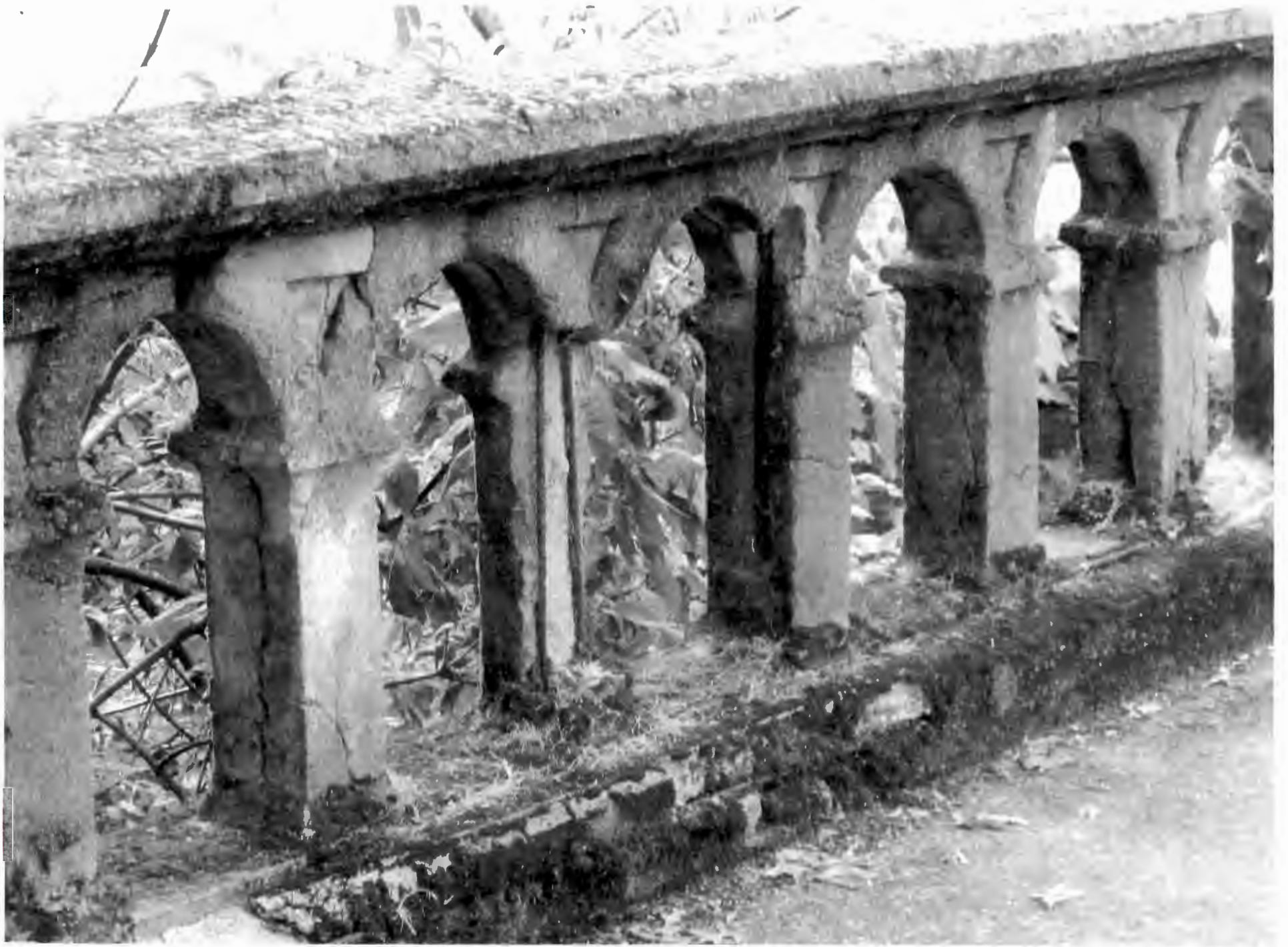
Deteriorating rail arches
