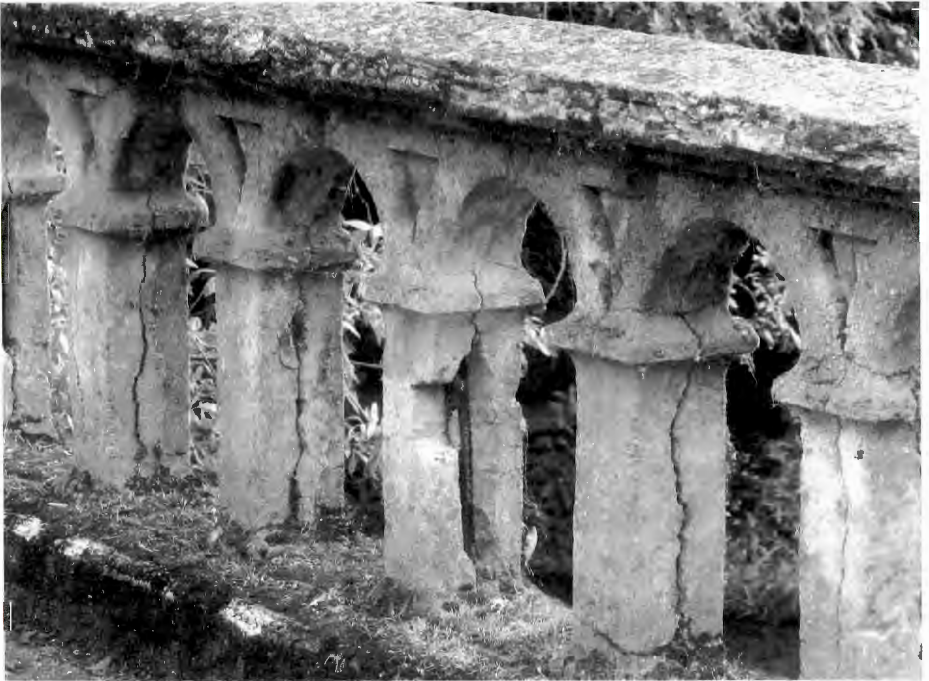
Deteriorating rail arches
