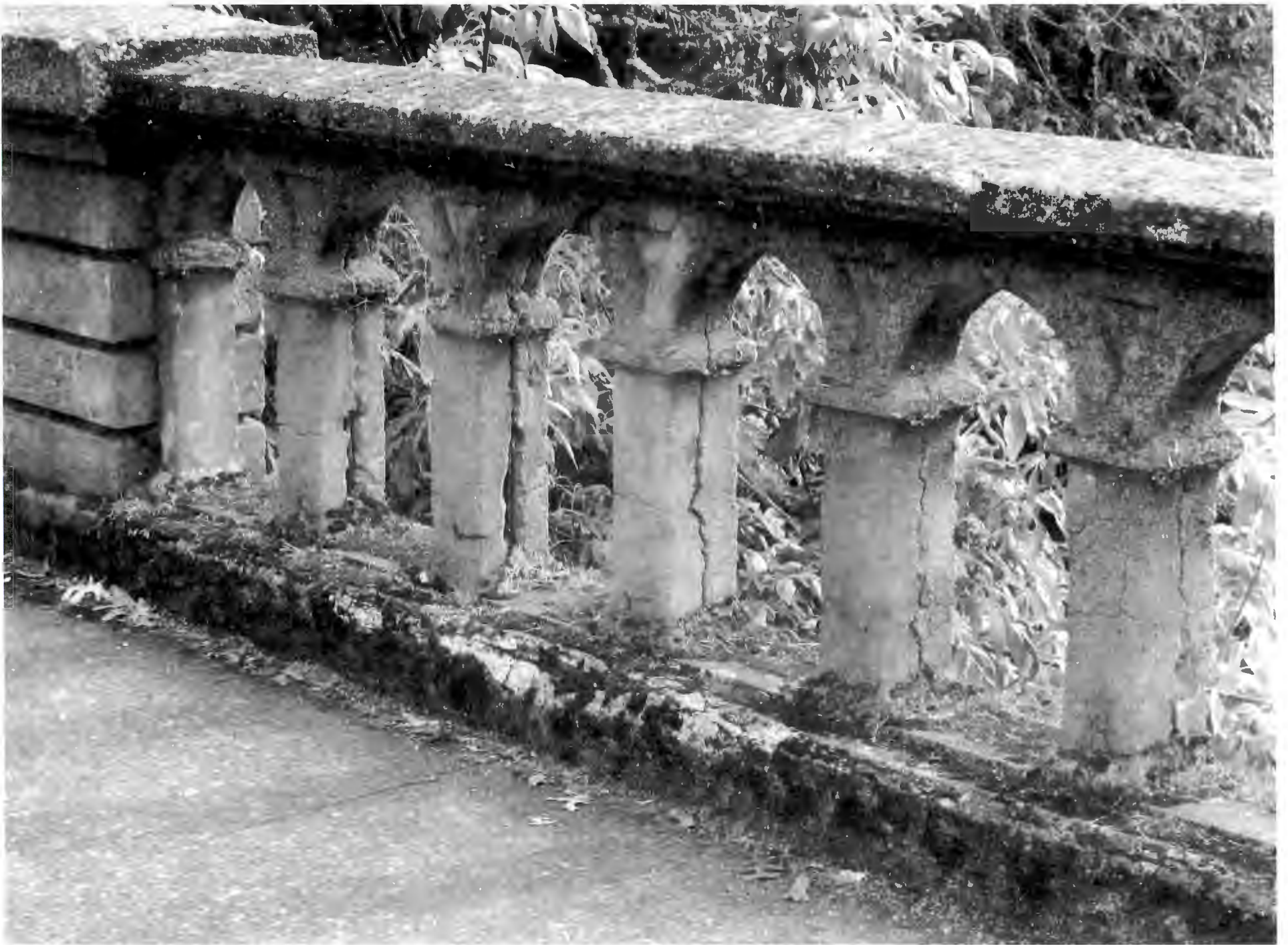
Deteriorating rail arches
