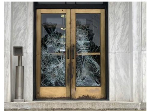
Below: Damage to Capitol doors. (photo courtesy of Willamette Week)
