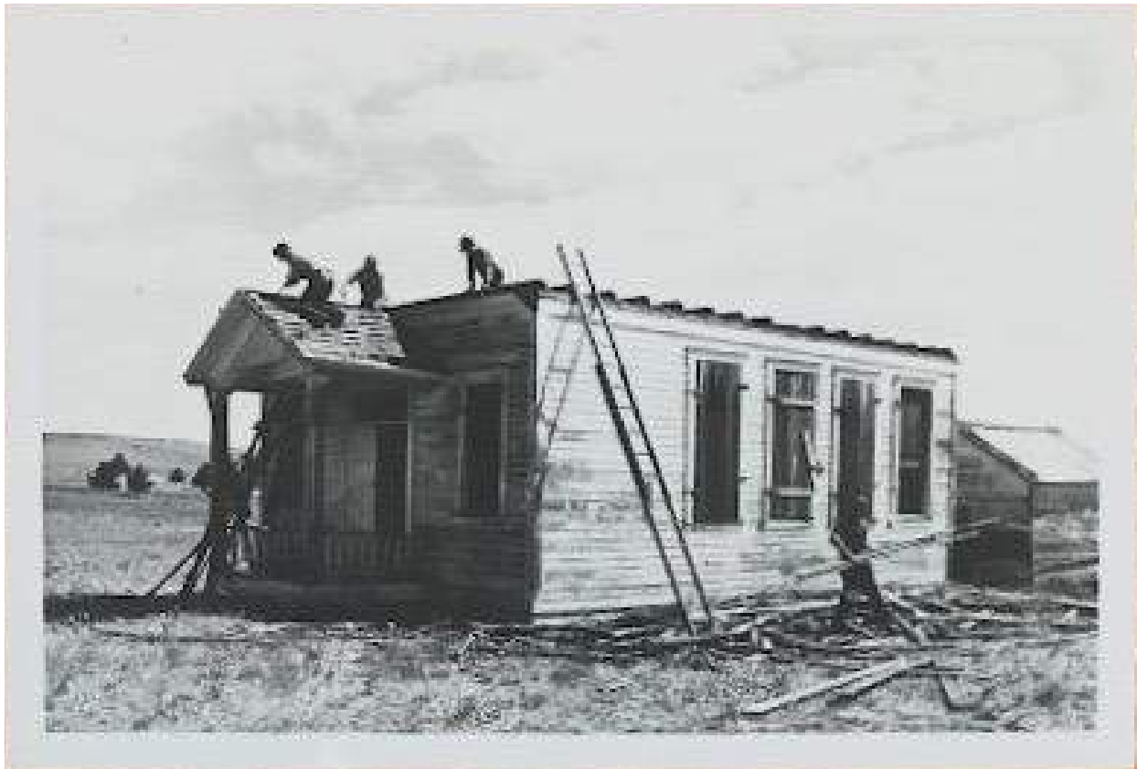
Image 5: Undated image of Criterion Schoolhouse with roof removed. Source: Criterion Schoolhouse Committee (Oregon State Fair Foundation) image collection.
